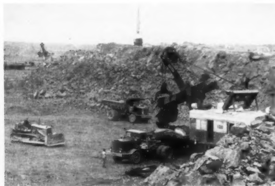
ORE PRODUCTION TEAM: Jet piercer, 6-yard electric shovel with 5-yard bucket, Diesel trucks, and cleanup Caterpillar.
